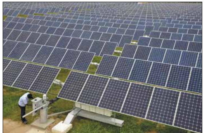
A one-megawatt solar plant goes online in Tamil Nadu. Photo: The Hindu
