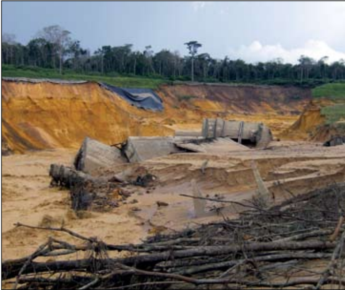
Site of Apertadinho Dam after it ruptured. Photo: Rondoniagora
