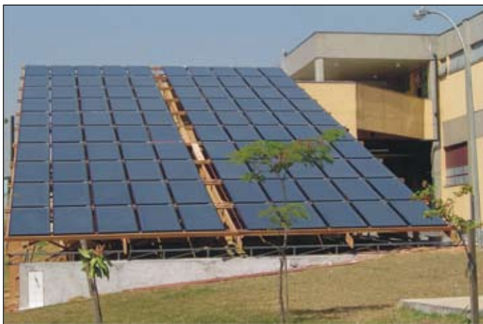
Solar installation at a São Paulo hospital.
