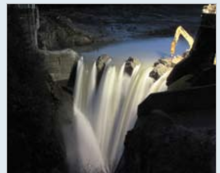
Removal of the Elwha Dam began in Washington state. Photo: National Park Service
