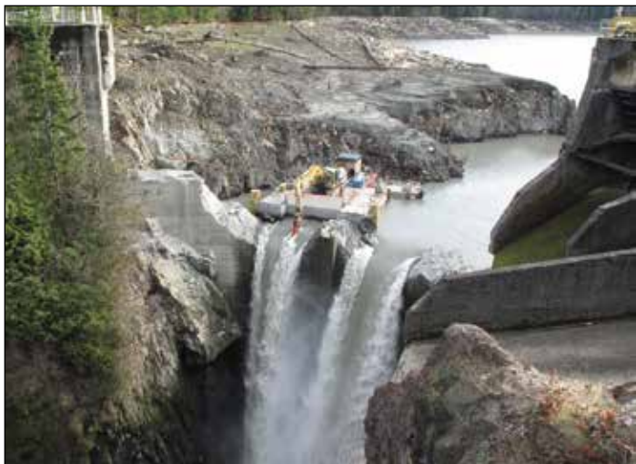
The top quarter of Glines Canyon Dam was removed from the Elwha River with a hydraulic hammer on a barge anchored upstream of the dam. Photo: National Park Service, courtesy Lower Klallam Tribal Library
