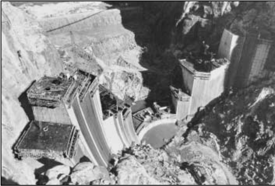
Cahora Bassa under construction. Since the site was a virtual fortress, combatants attacked powerlines instead.
