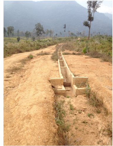
Poorly built and planned
