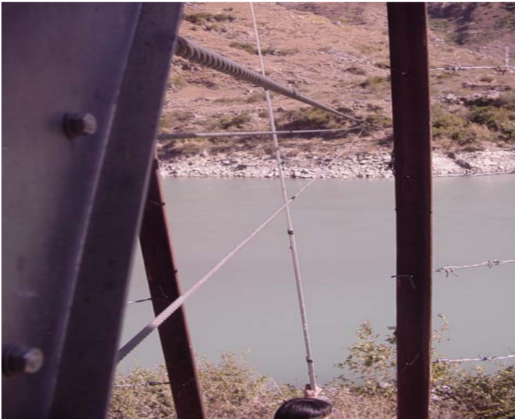
Figure 5.1: Cableway system installed at Punatsangchhu River. (Department of Energy, 2009)
