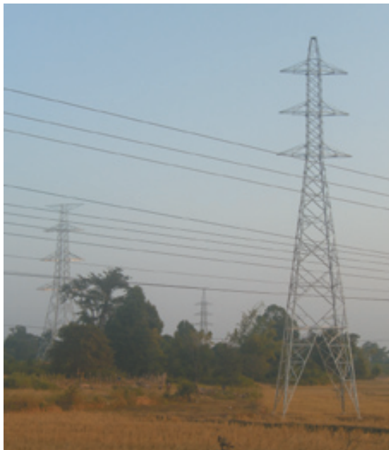
High voltage transmission towers for Nam Theun 2. Photo: Shannon Lawrence
