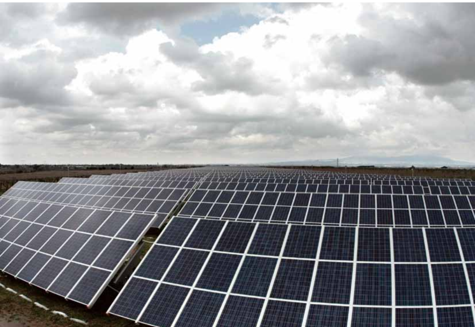
Solar Panels. Photo: Statkraft
