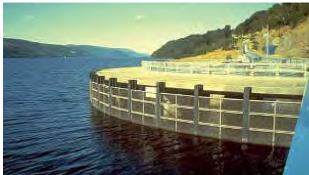
Figure 6-13: Example of fish screens at hydropower intakes.
