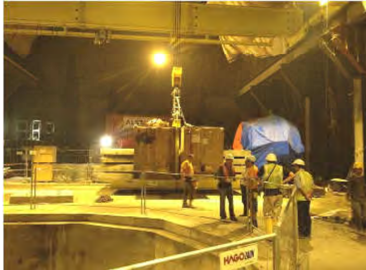
Figure 2-10: The powerhouse under construction at Dagachhu; Nikachhu will have a similar configuration.
