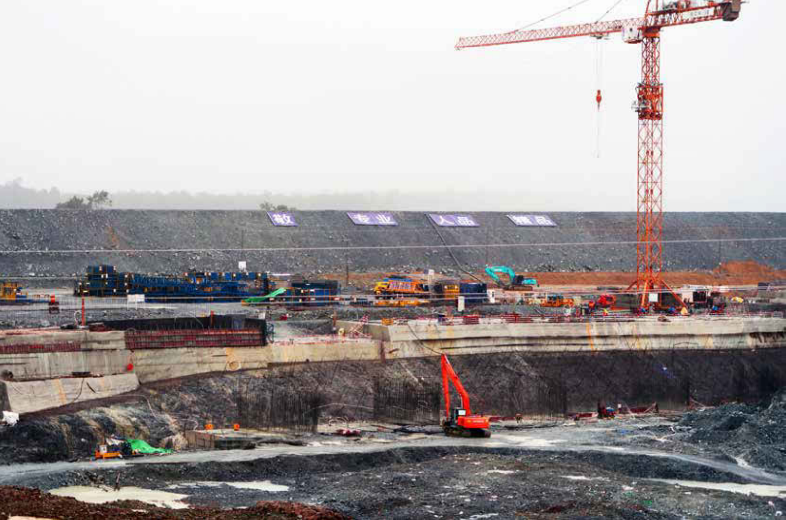
Photo © Prachatai 2015. CAMBODIA - Lower Sesan II Dam. Re-printed under a Creative Commons Attribution License.
