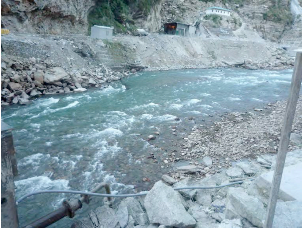
Photograph of dumping in riverbed with gabion retention walls on opposite bank crumbling
