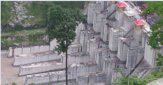
Construction of Teesta V Dam, Sikkim, India, 2008. Photo by Samir Mehta, International Rivers.
