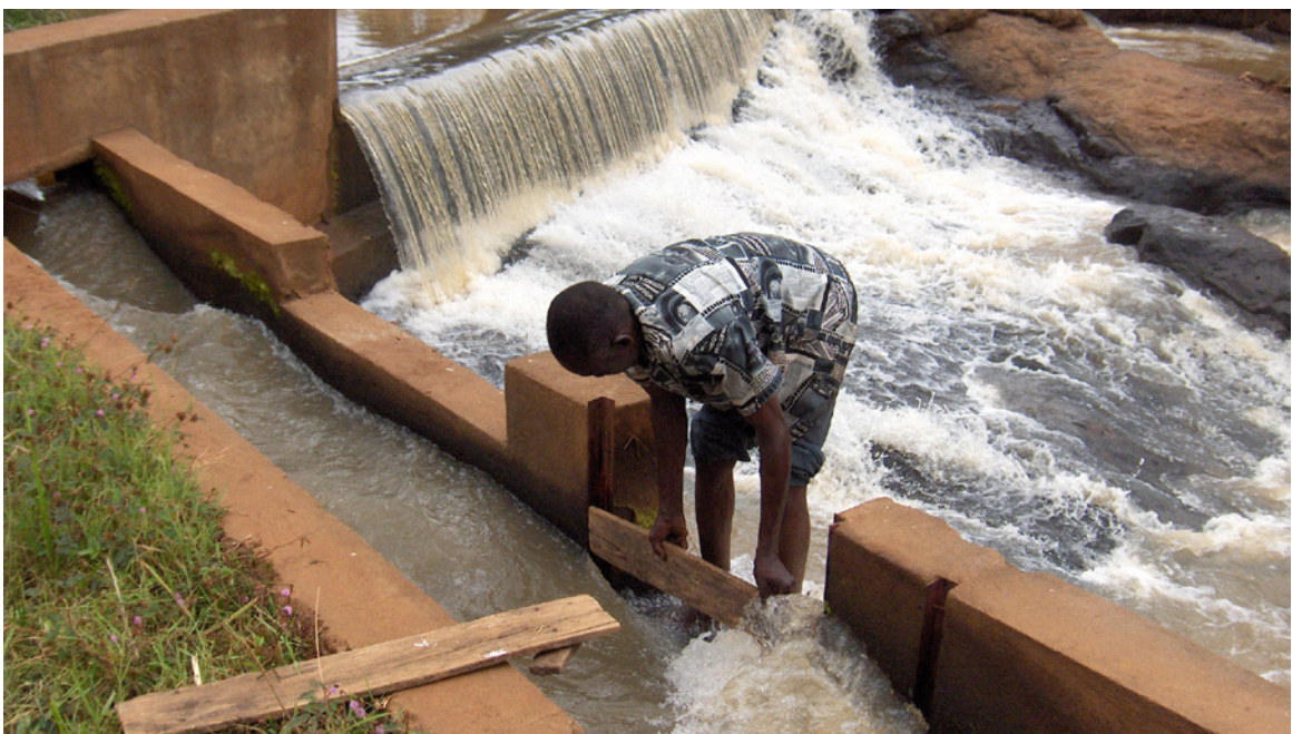
Opening the sluice gate on a small hydro project in Africa. Photo: Wim Klunne
