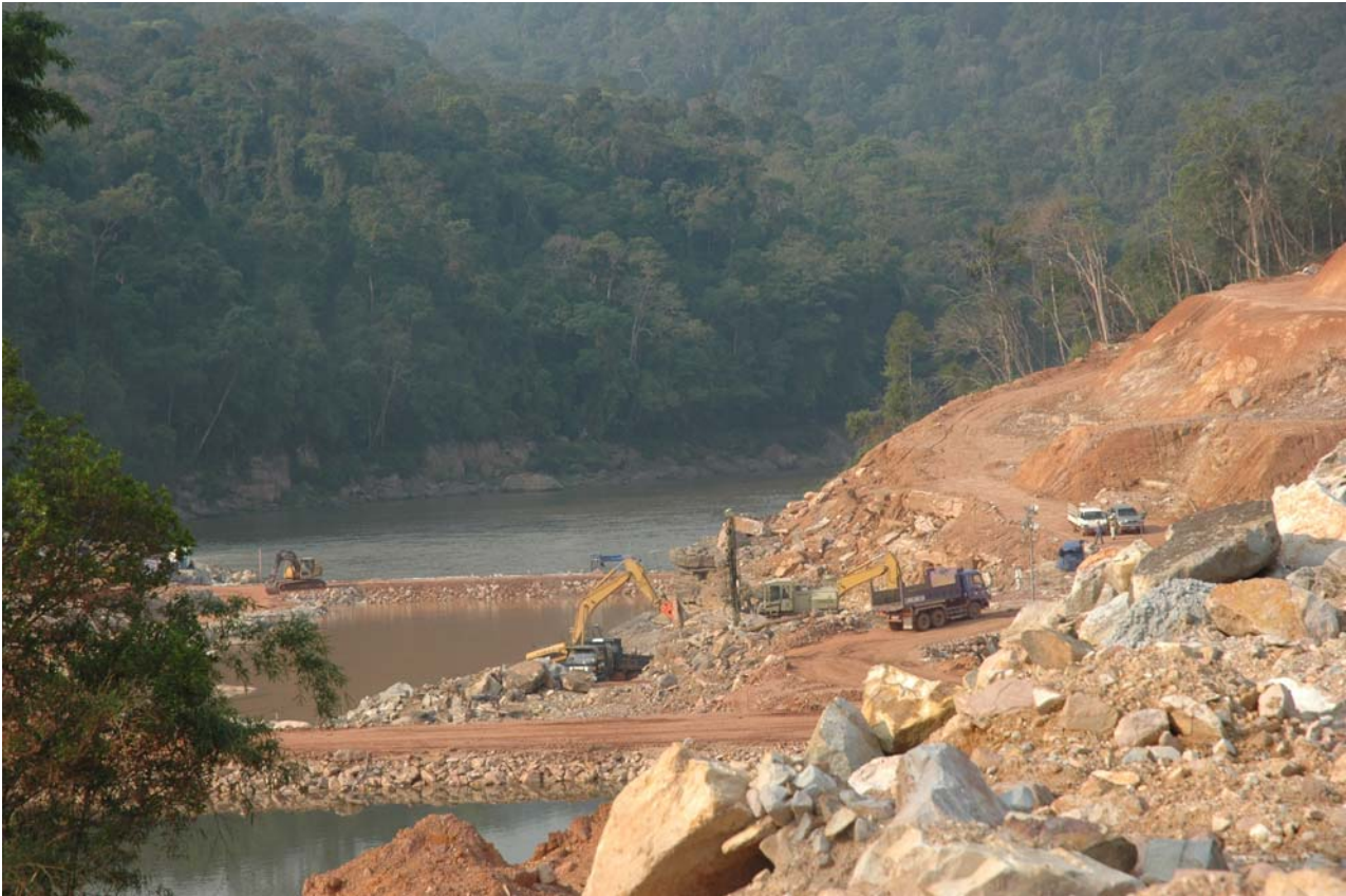
The Nam Thuen 2 dam, under construction on the Nam Theun River, central Laos.
